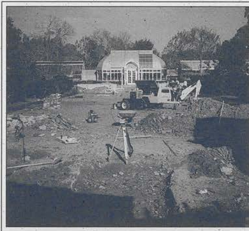
FALL 1996, THE JAPANESE CEDARS HAVE BEEN REMOVED, RECONSTRUCTION OF GARDEN WALLS IN PROGRESS.
