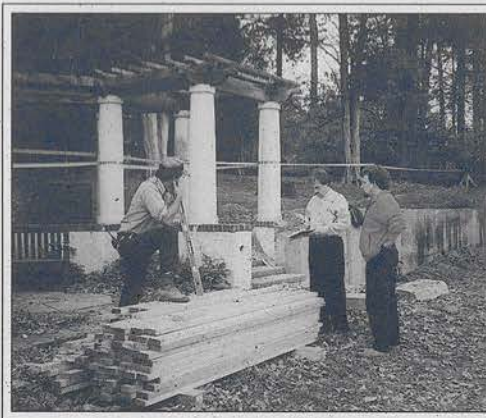
FROM LEFT: RICK CATES AND JED DANIEL OF SEAGER WATERPROOFING INC. DISCUSS THE WALL PROJECT WITH A. CHESTER "CHET" THOMAS, ASLA OF THE JAEGER COMPANY.
